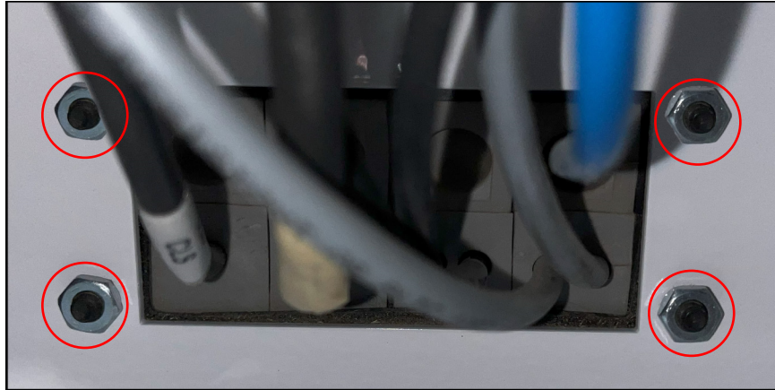
Figure 7: Grommet Bracket Nuts on Enclosure Side
