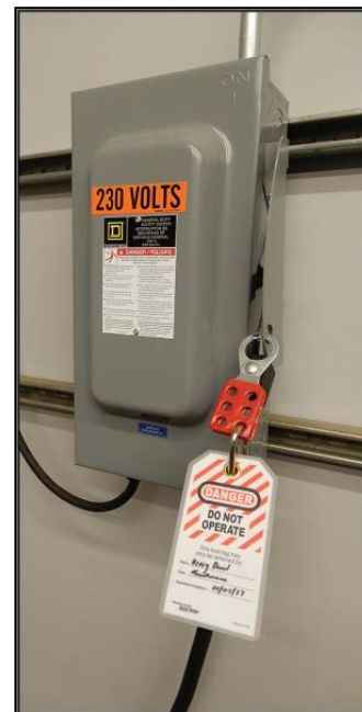
Figure 1: Lockout/Tagout on the Power Source Panel
