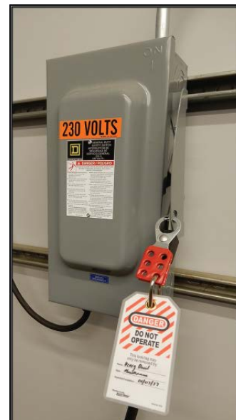
Figure 1: Lockout/Tagout on the Power Source Panel
