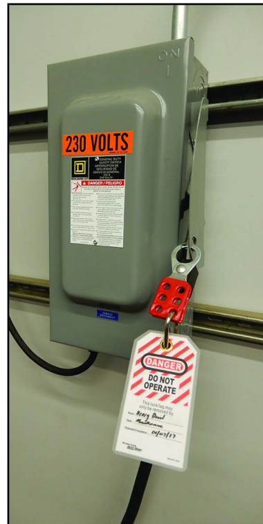
Figure 1: Lockout/Tagout on the Power Source Panel
