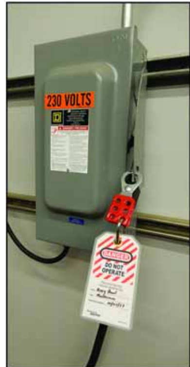
Figure 1: Lockout/Tagout on the Power Source Panel
