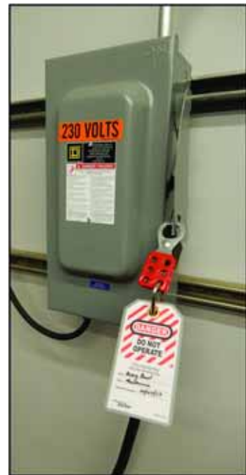
Figure 1: Lockout/Tagout on a Power Source Panel
