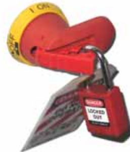
Figure 1: Lockout/Tagout on the Main Electrical Enclosure
