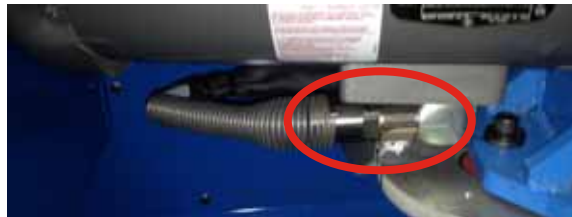
Figure 7: Connection Point at Saw Blade Motor
