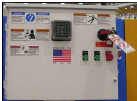
Figure 2: Lockout/Tagout on the Main Electrical Enclosure
