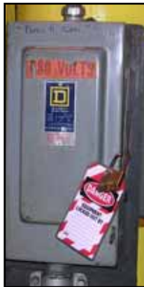
Figure v-2: Lockout/Tagout on the Power Source Panel
