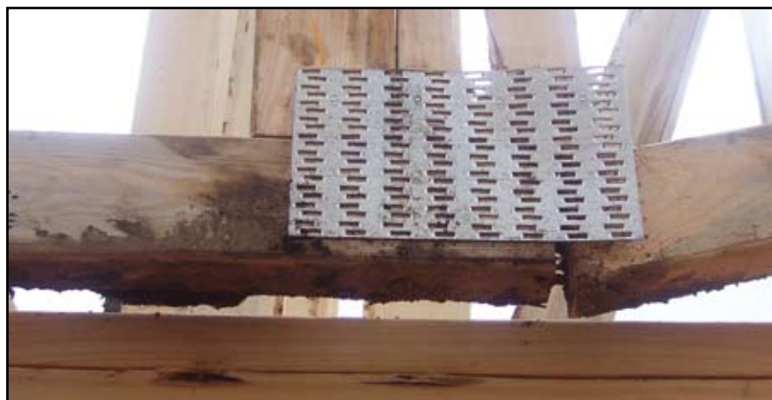
Figure 1: A typical damaged joint. Notice the connector plate teeth have pulled out of the lumber on the right side of the joint, and one web is split along the grain. Also, note the mud on the lumber, a consideration when using adhesives.
