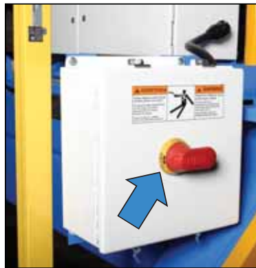
Figure 3: Disconnect Switch to Lockout/Tagout
