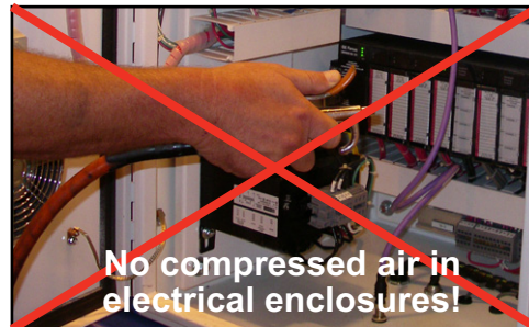
Figure 6-3: Never Use Compressed Air Inside an Electrical Enclosure
