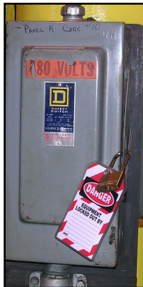
Figure 2-3: Sample of a Lockout/Tagout Mechanism on a Power Source Panel
