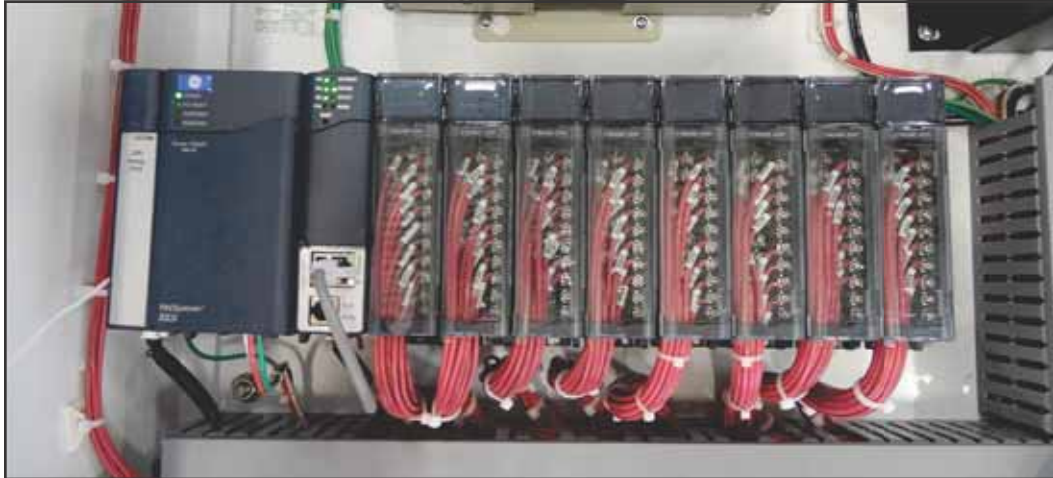
Figure 6-3: PLC in Main Electrical Enclosure
