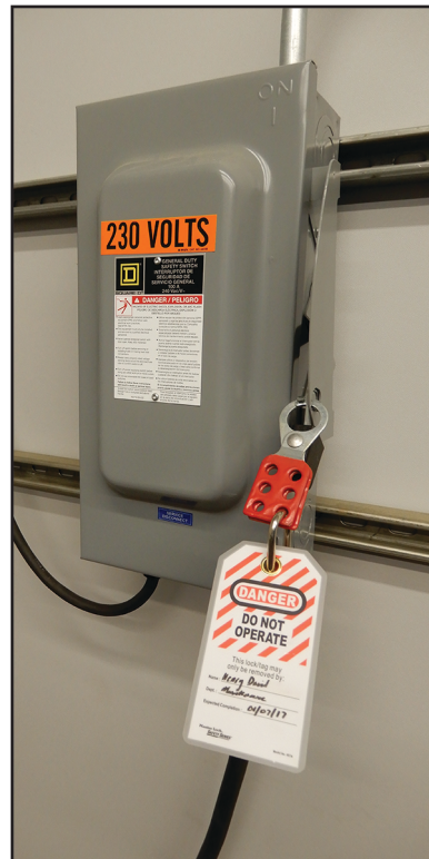
Figure 2: Lockout/Tagout on the Power Source Panel
