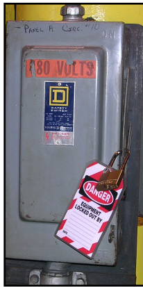
Figure ii-2: Lockout/Tagout on the Power Source Panel
