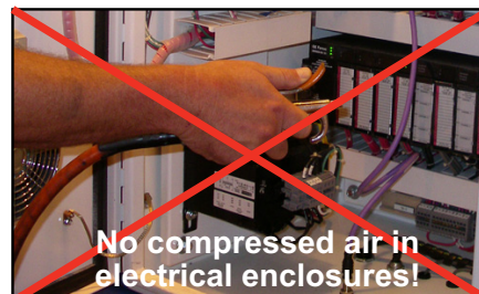
Figure 7-5: Never Use Compressed Air Inside an Electrical Enclosure
