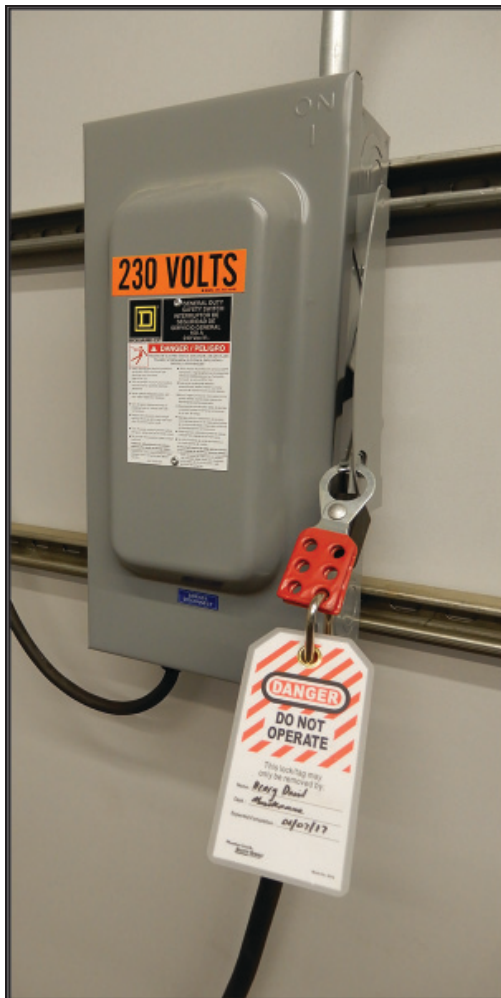
Figure SAFETY-2: Lockout/Tagout on the Power Source Panel
