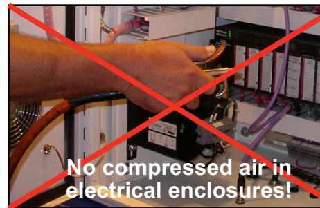
Figure A-1: Never Use Compressed Air Inside an Electrical Enclosure
