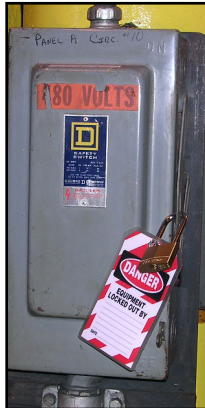
Figure SAFETY-3: Sample of a Lockout/Tagout Mechanism on a Power Source Panel
