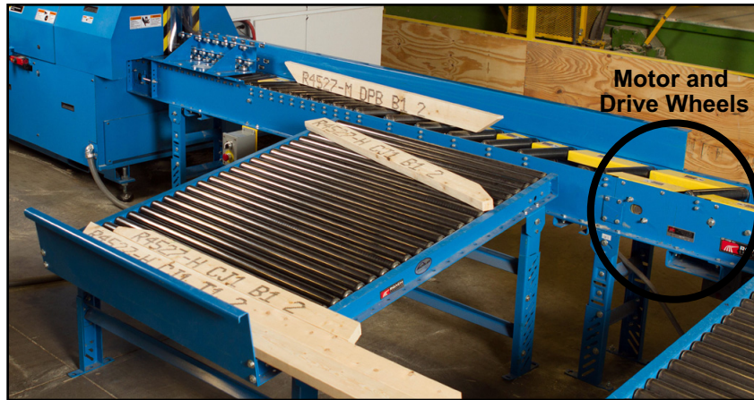
Figure 2-51: Powered Skewed Conveyor Maintenance
