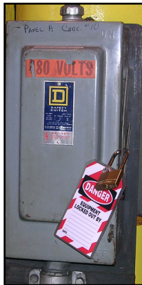
Figure IV-2: Lockout/Tagout on the Power Source Panel
