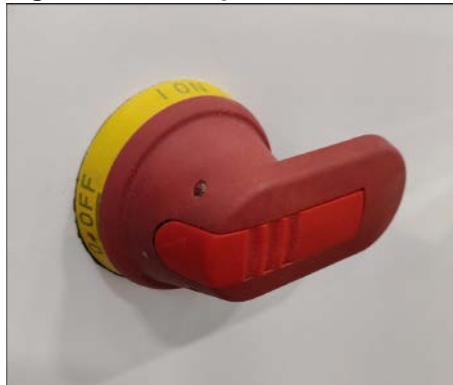
Figure 1-1: Example of a Disconnect Switch in Off Position
