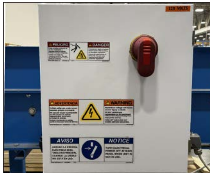
Skewed Conveyor Disconnect Switch
