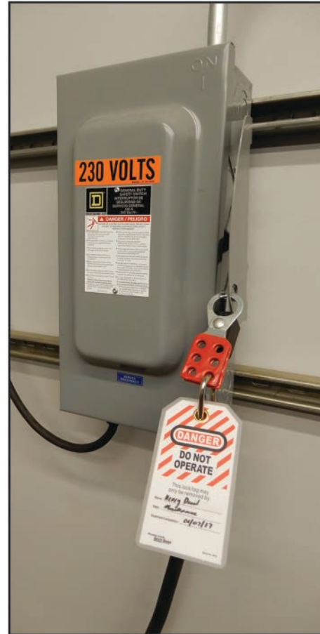
Figure 1-3: Sample of a Lockout/Tagout Mechanism on a Power Source Panel
