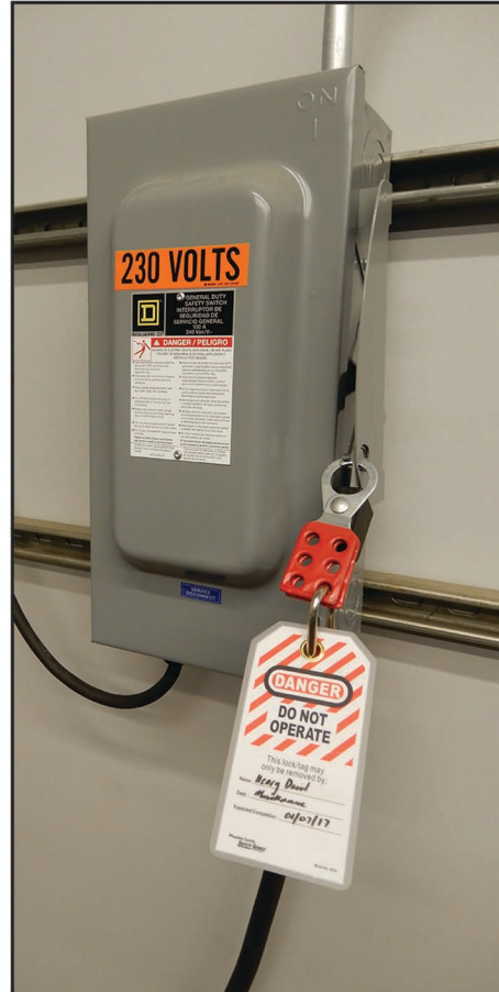
Figure 1-1: Sample of a Lockout/Tagout Mechanism on a Power Source Panel
