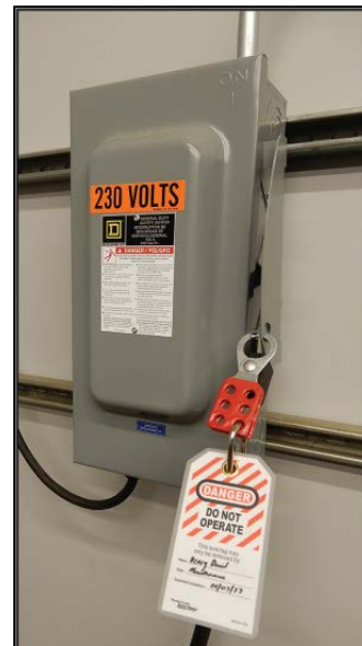
Figure 1: Lockout/Tagout on the Power Source Panel
