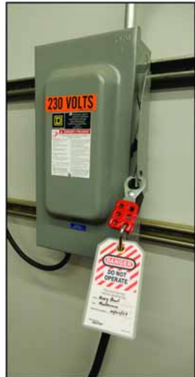
Figure 1: Lockout/Tagout on the Power Source Panel
