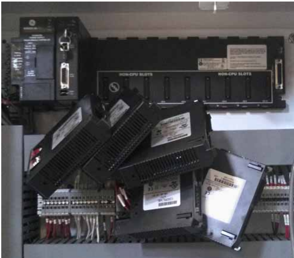
Figure 9: Modules and I/O Expansion Cable Disassembled from PLC Rack
