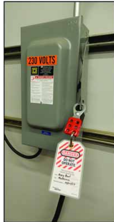
Figure 1: Lockout/Tagout on the Power Source Panel
