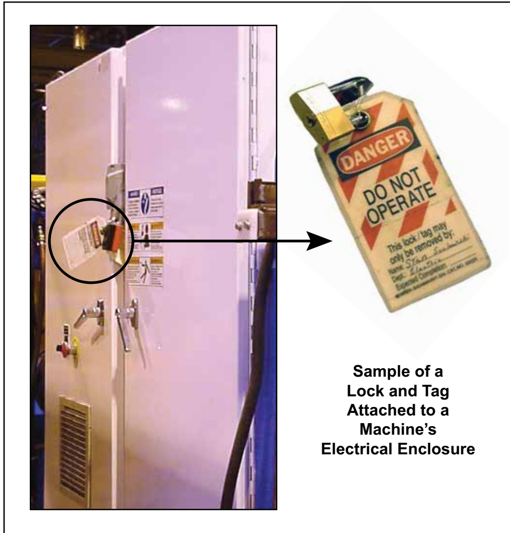
Figure 1: Lockout/Tagout on the Main Electrical Enclosure
