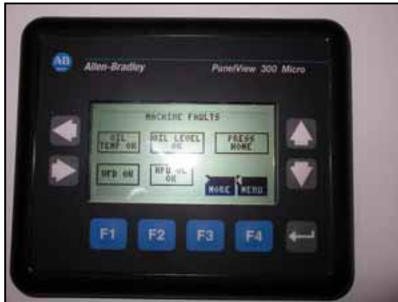
Figure 6-5: Control Display Showing the Machine Faults Screen
