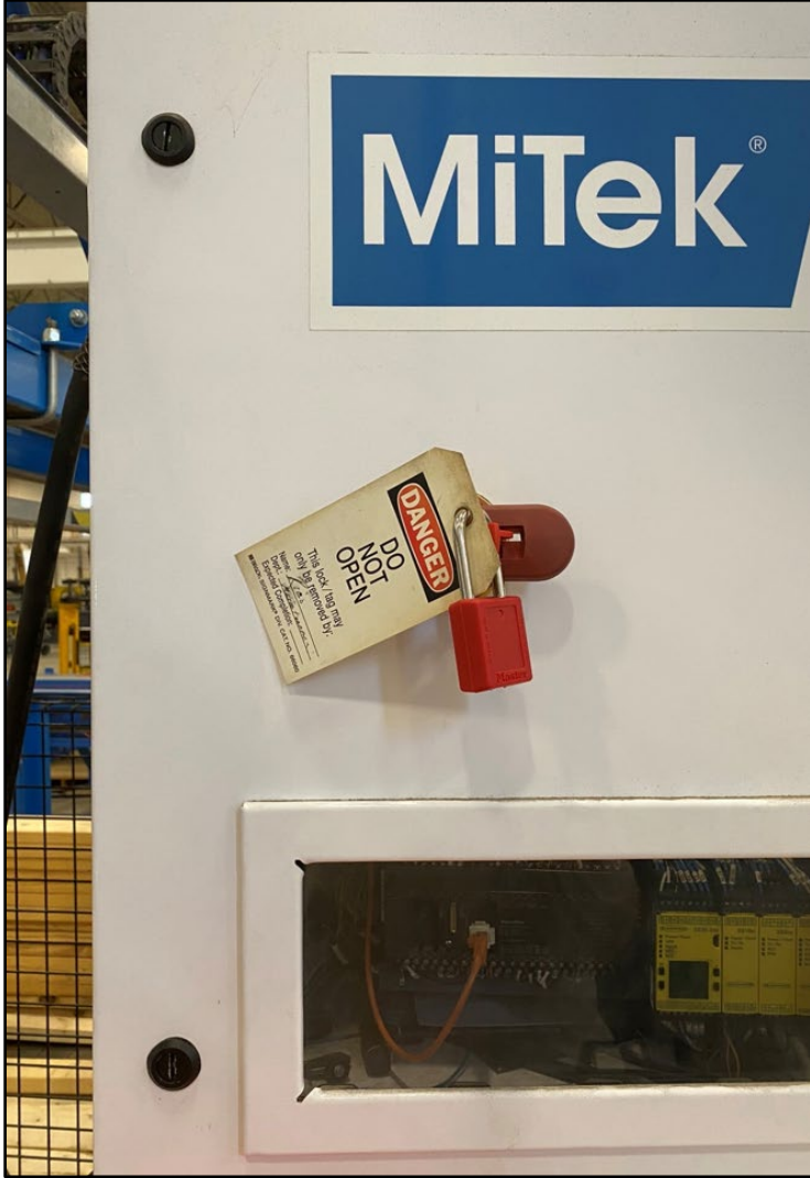
Figure 1-2: Sample of a Lockout/Tagout Mechanism on an Electrical Enclosure
