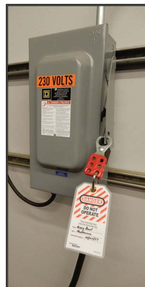
Figure 2: Lockout/Tagout on the Power Source Panel
